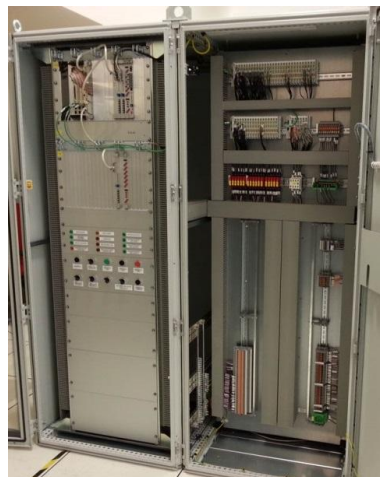
Control System Replica
